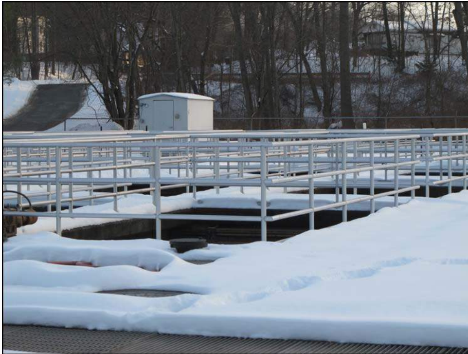
Photo 9: Settling tanks at WWTF.
