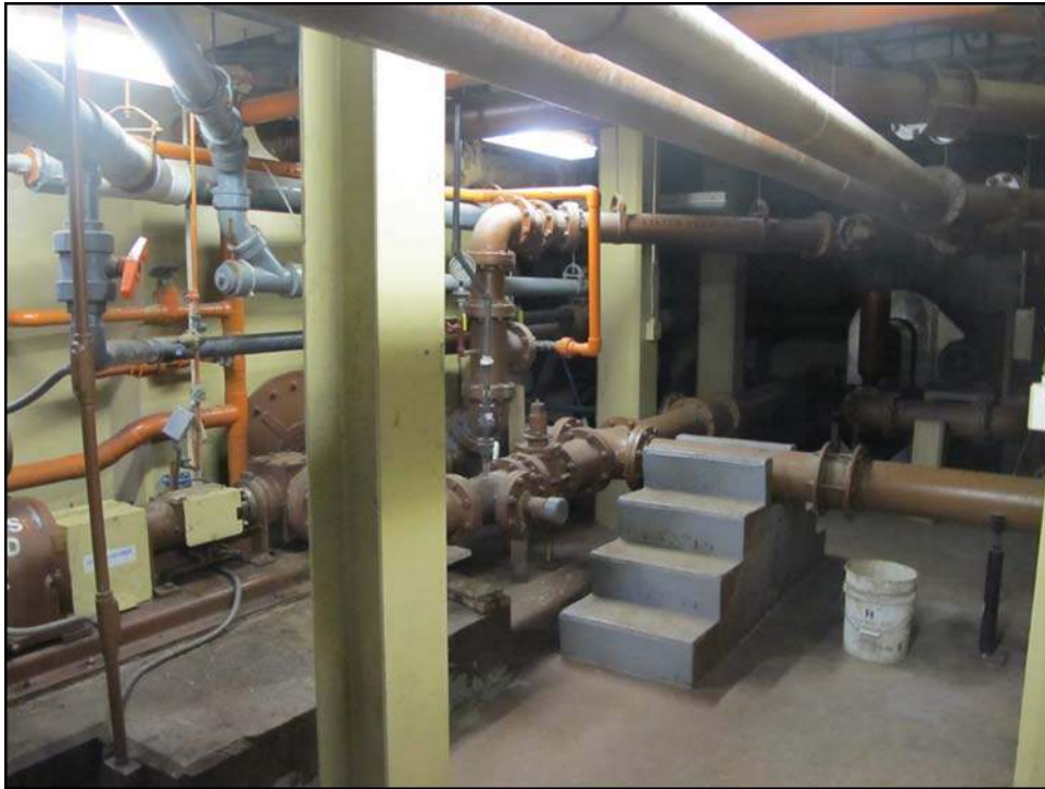
Photo 13: Piping network in the main operations building.
