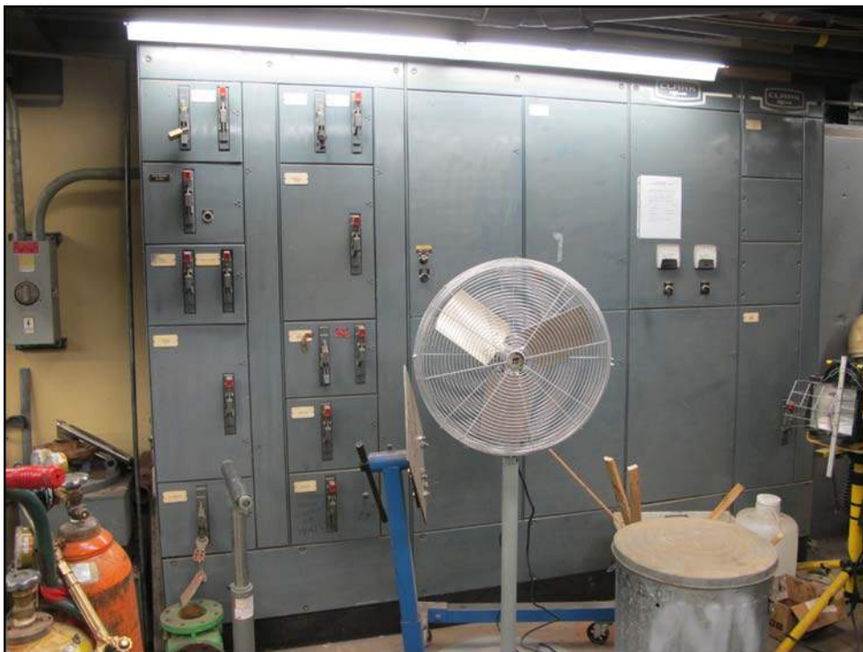
Photo 12: Main electrical panel. Likely interconnection point.
