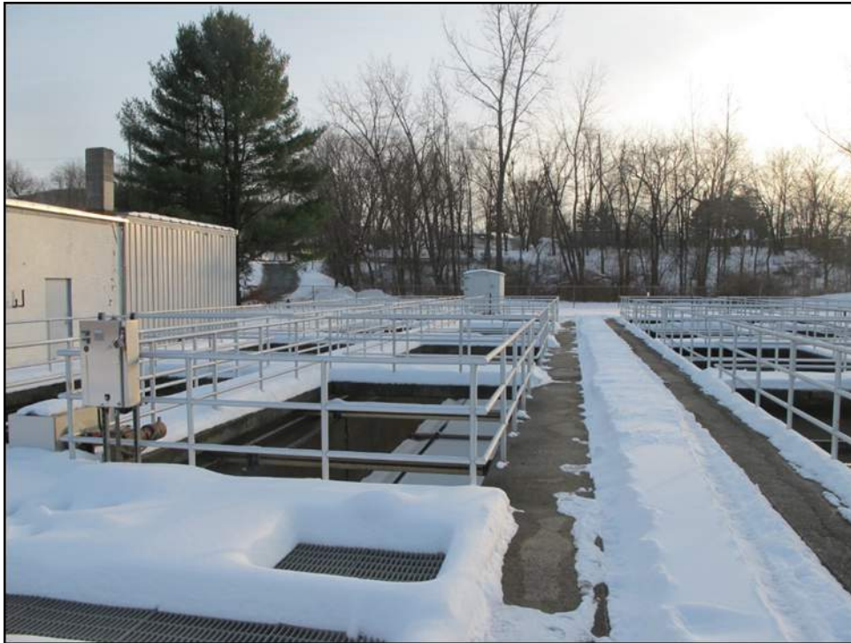
Photo 11: Settling tanks at the WWTF.
