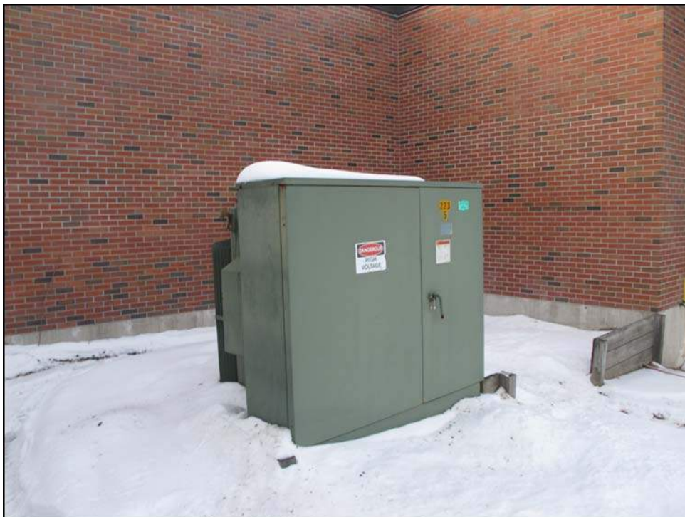
Photo 8: Main electrical transformer to facility.
