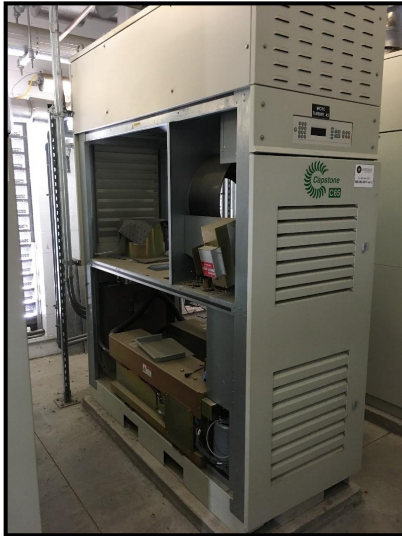
Figure 1-5: Photo of Decommissioned Microturbine #2
