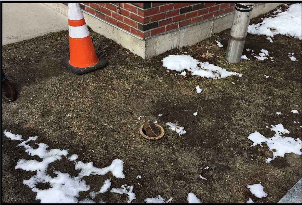
Figure 1-4: One of the Valves Used to Manually Bleed Moisture from the Digester Gas
